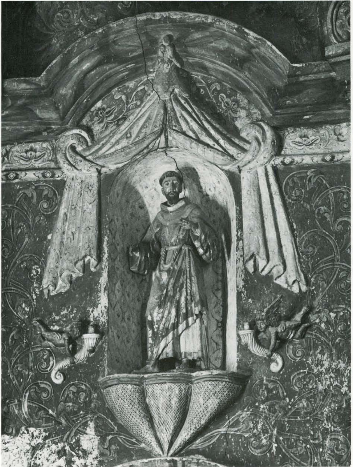
Figure 26. Statue of St. Francis of Assisi at San Xavier Mission. Note crack in the wall behind the statue, caused by the 1887 earthquake (A16). Photo courtesy of John P. Schaefer.
